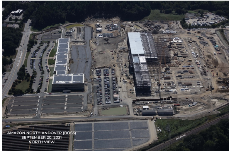
Fig. 2. North Andover Amazon Robotics Sortation Facility, 1600 Osgood Street. Construction as of September 2021.
